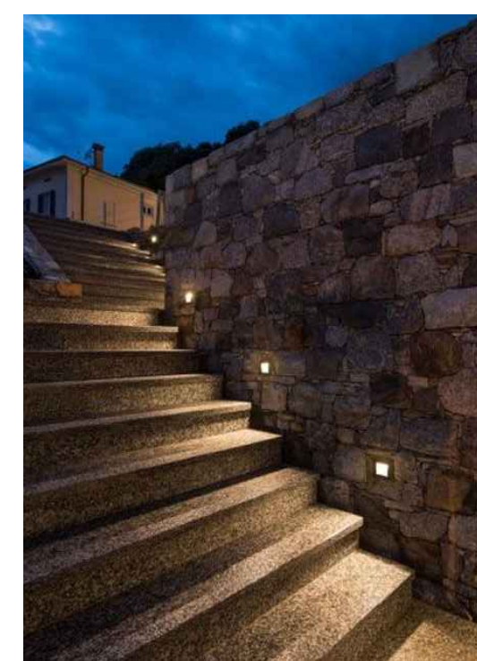
Building mounted light
